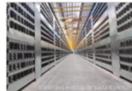
EXISTING PHOTO OF DATA CENTER
